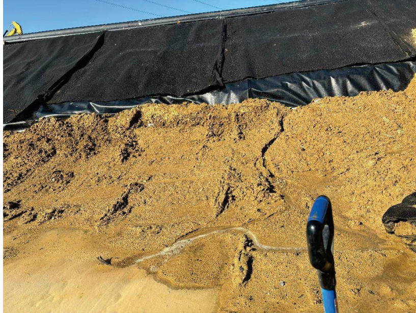
Photograph 1. View of upland (active construction area) at wetland determination sample point SP01. Photograph taken facing west.
