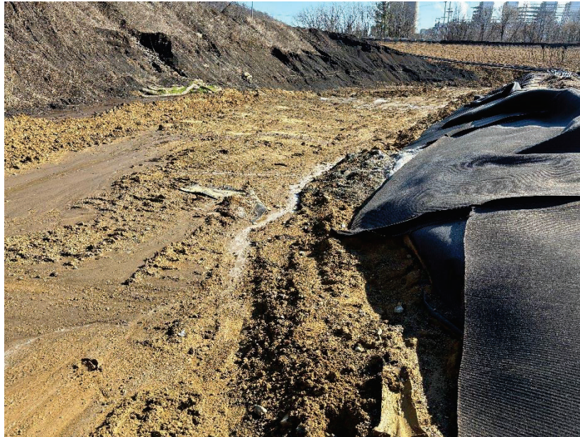
Photograph 3. View of upland (active construction area) at wetland determination sample point SP02. Photograph taken facing northeast.
