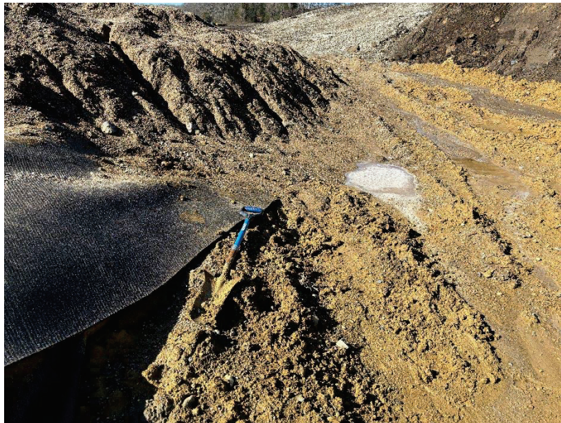
Photograph 4. View of upland (active construction area) at wetland determination sample point SP02. Photograph taken facing west.
